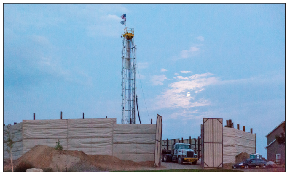
Above: Drilling by the Woodmoor Water and Sanitation District for Well 21 at Alexandria Drive and Hammock Oaks Court in the Misty Acres subdivision began Aug. 20 and will continue around the clock until completion in two to three weeks. The drilling must be done continuously until complete to prevent the well shaft from collapsing. The site is surrounded by 16-foot sound barriers. Landscaping will be done at the well site when drilling is complete. In addition to the construction at the well site, a pipeline will have to be installed to transport the water from the new well to a processing facility. Residents in the pipeline corridor will be notified. The total budget for the project is $2 million. Photo by Jackie Burhans.
