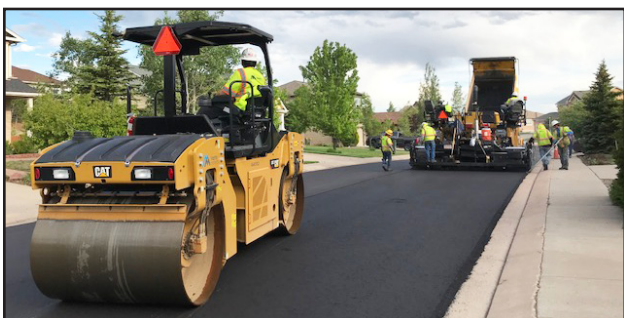
Above: Triview Metropolitan District contracted with Martin Marietta to fulfill overlay work in specific neighborhoods as part of its 2019 road overlay project. The expected completion date for the entire project was June 27. Photo by Natalie Barszcz.
