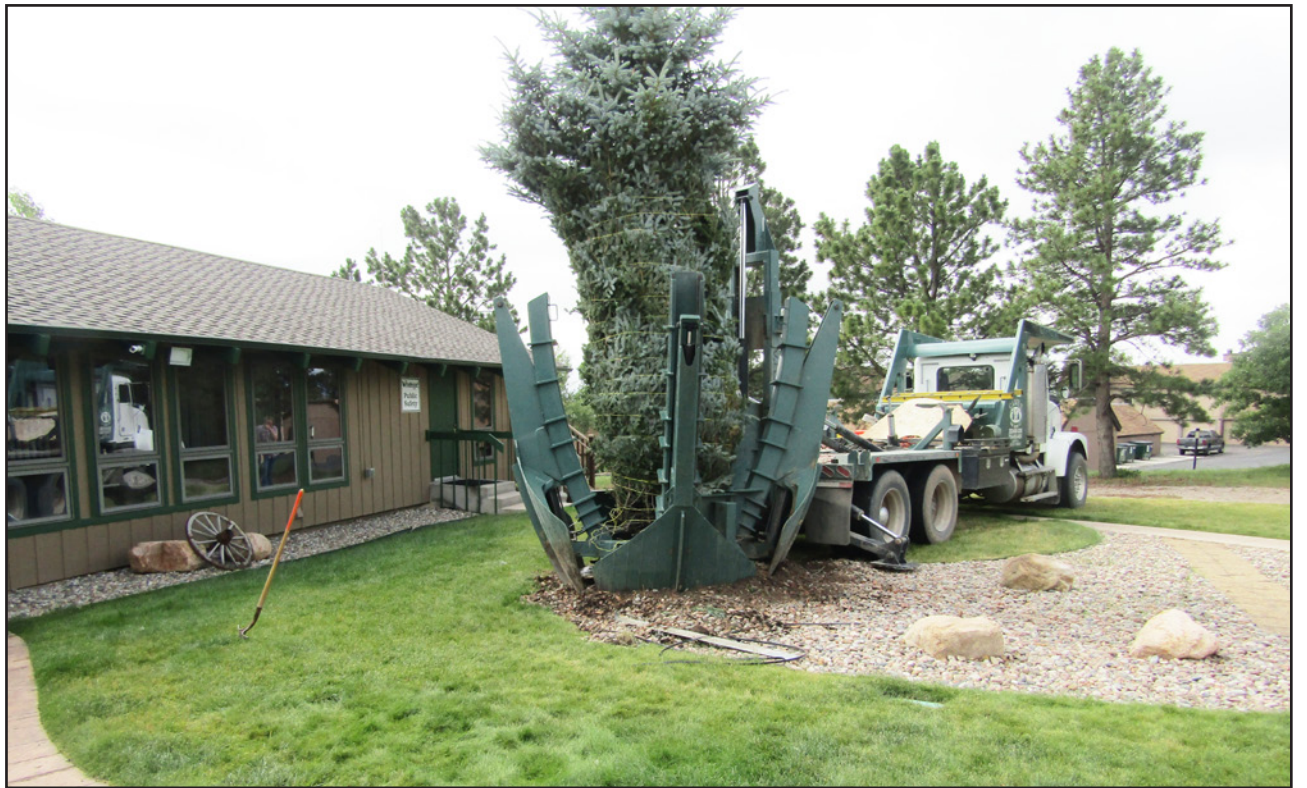
Above: A large blue spruce was successfully moved before beginning excavation for the Woodmoor Public Safety expansion at The Barn. Photo courtesy of WIA.
